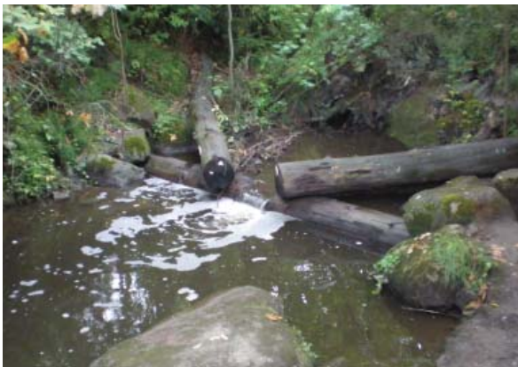
Restoration work at Upper Springbrook Creek will include placement of large woody debris
